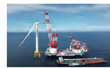
三峡新能源大连市庄河海上风电场项目 Three Gorges New Energy Dalian Zhuanghe Offshore Wind Farm Project
